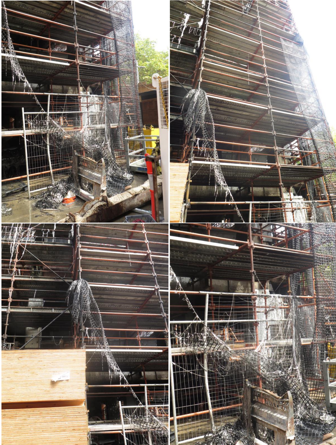
As fire ascended and progressed through the scaffold containment mesh, the material forming the mesh lost strength and failed, allowing large sections of burning high-density polyurethane to separate and fall, igniting new fires. There were three problems with the scaffold containment mesh; fire ascended the mesh, fire travelled sideways and fire “dropped down” ignited new fires on lower levels.
